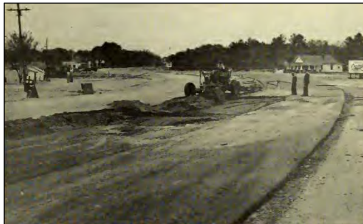
Figure 5. Original caption reads “Among the new primary road projects under construction this summer is a face lifting job for US 70 between Raleigh and Clayton” (source: North Carolina Roadways 1951)
