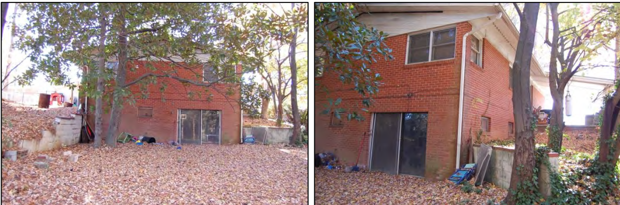
Figure 88. Garner Animal Hospital: house’s north rear elevation, at left, and north rear and west side elevations, at right
