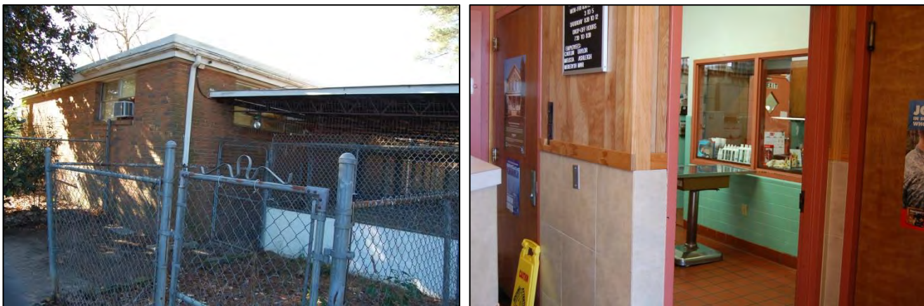
Figure 86. Garner Animal Hospital: east side and north rear elevations, at left, and lobby and green-tiled examination room, at right
