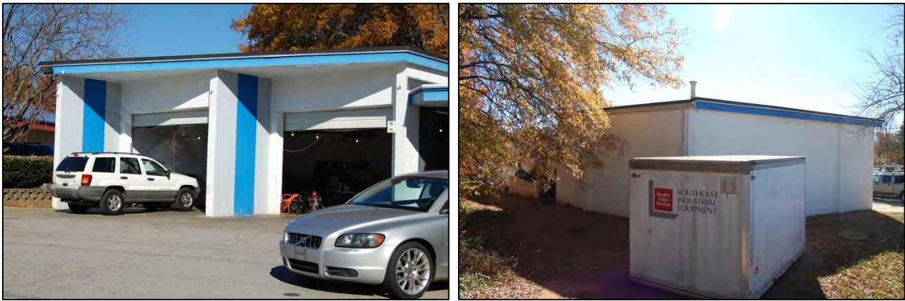
Figure 51. Looking northwest at service bays, at left, and southeast at blank side and rear walls, at right
